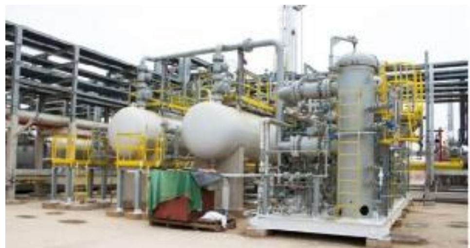
Atuabo Gas Processing Plant
